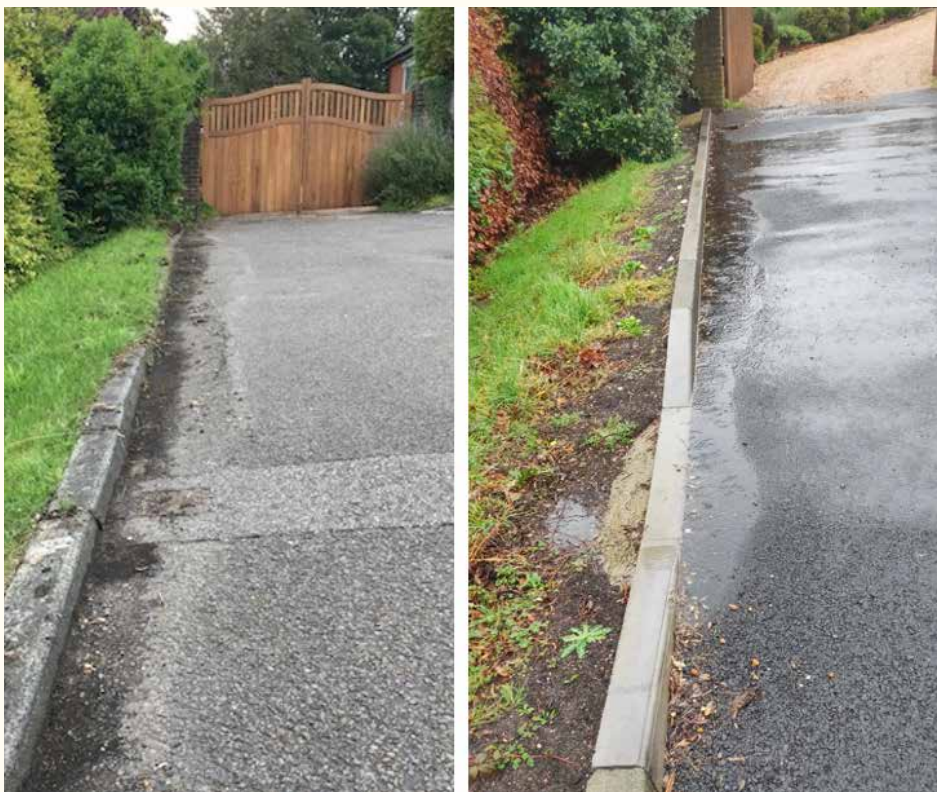
Dropped kerbs to manage surface water on the Cuilfail Estate, Lewes. Image: OART
