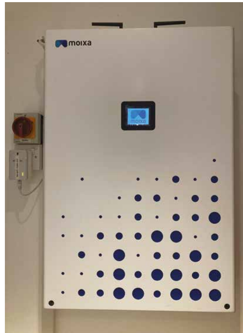
Wall mounted solar battery
