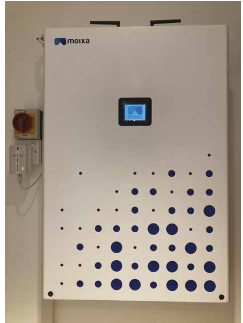
Wall mounted solar battery
