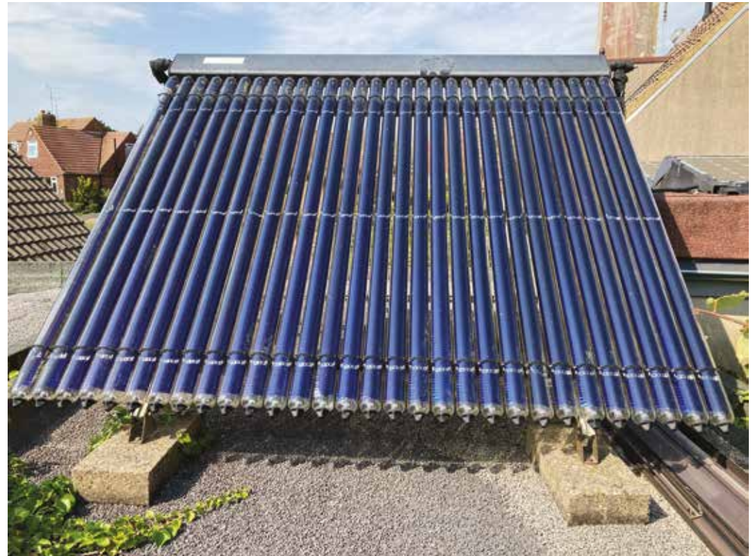
Solar thermal panel
