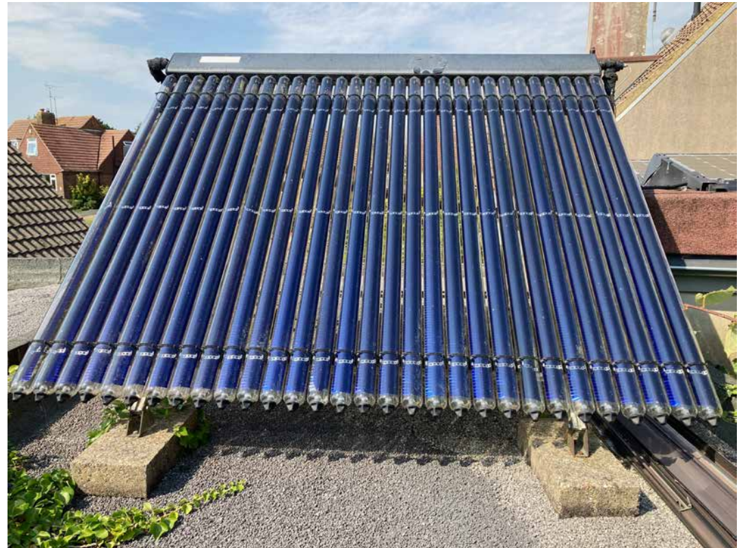
Solar thermal panel
